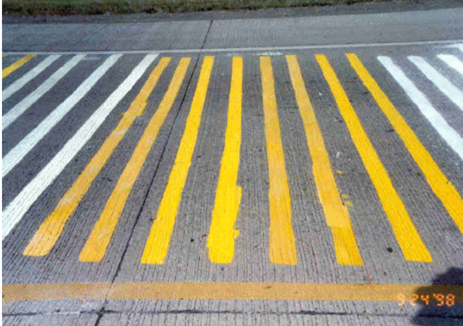
Photo 5 - Final eight test stripes on concrete test section. Four white latex E-2706 stripes (left side). Four white latex E-3427 stripes (right side).
