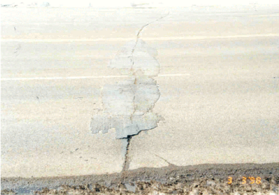
Photo 6 -- Poly-patch material missing---Probably by snowplows rapidly, adhesion could
