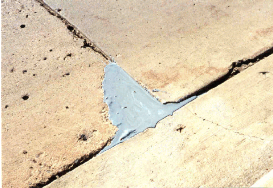
Photo 12 -- Typical spall filled with cold weather repair material
