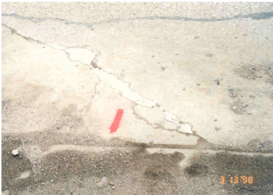
Photo 14 -- Warm weather repair material ---good condition
