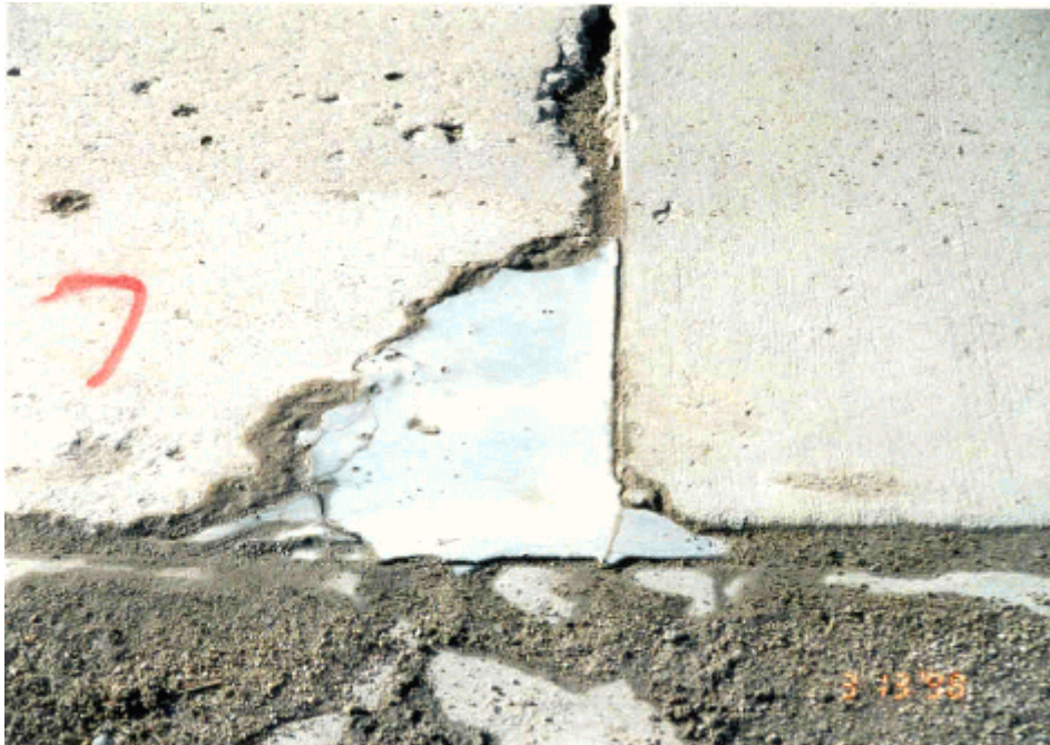
Photo 16 -- Cold weather repair material ---some cracking
