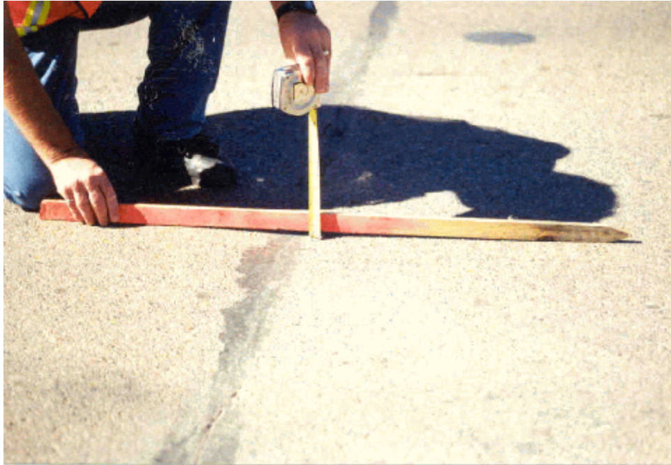
Photo 1 -- Transverse crack depression (Approx. ½")
