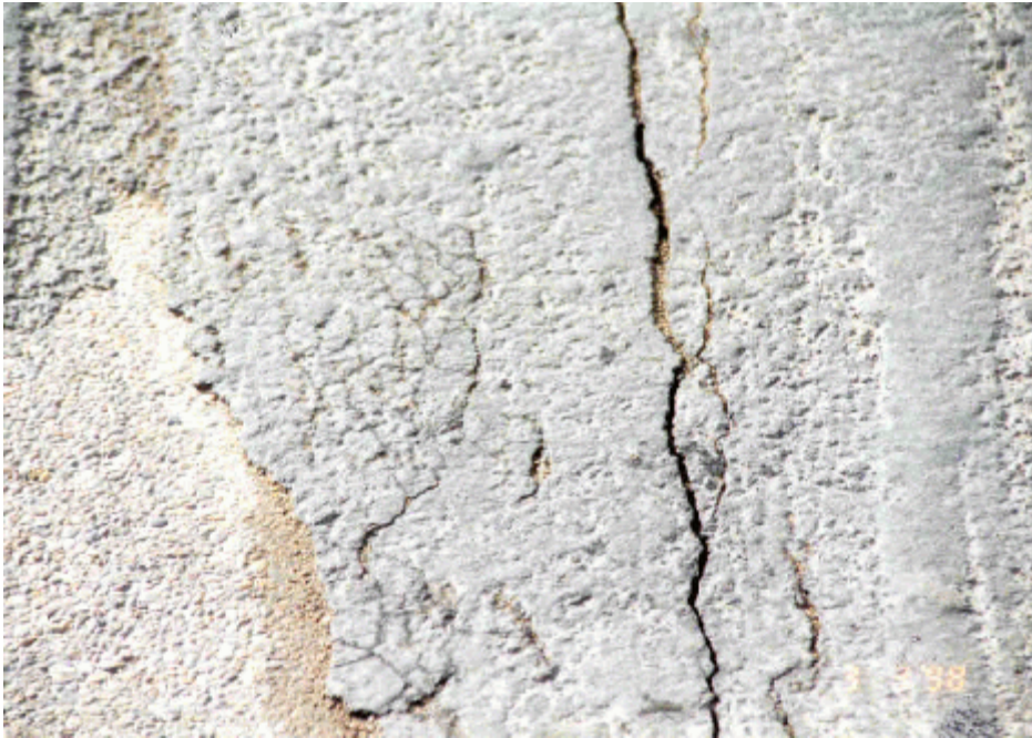
Photo 7 -- Small cracks developing in poly-patch material
