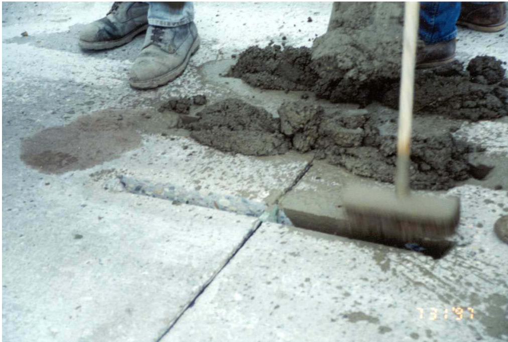
Photo 9 - View of the grout being applied to the dowel bar retrofit slot.
