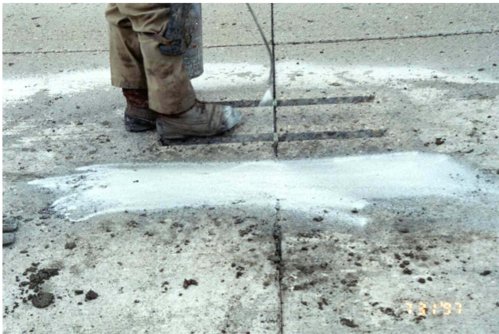
Photo 12 - View of the oil based curing compound being applied to the finished and grouted 3U18 patch mix.
