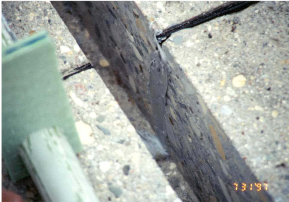
Photo 4 - Close-up view of the joint after the caulking is finished. and photo 5 shows the core board fabrication process.
