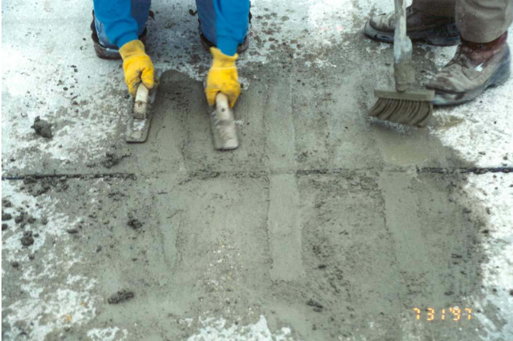
Photo 11 - View of the grout being applied to a finished 3U18 patch mix.
