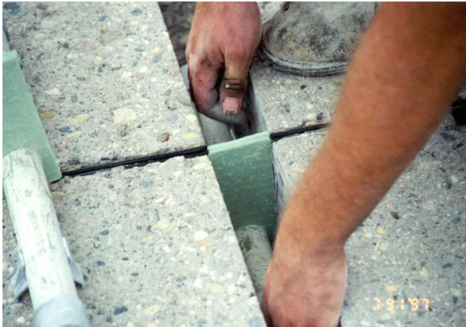
Photo 6 - View of the dowel bar and core board installed in the slot prior to the mix being placed.
