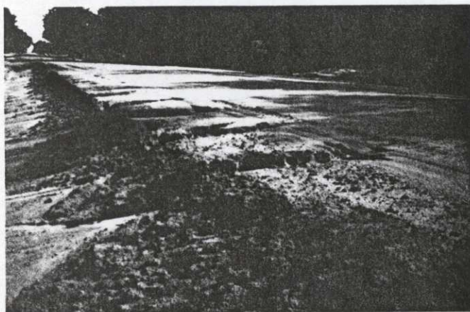
Another example of the CONSOLID™ System's stabilized base versus the untreated shoulder.
