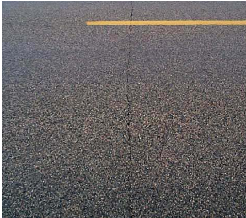
Photo 14 - Typical transverse crack.
