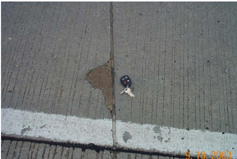
Photo 19 - Attempted spall repair in sealed control section.
