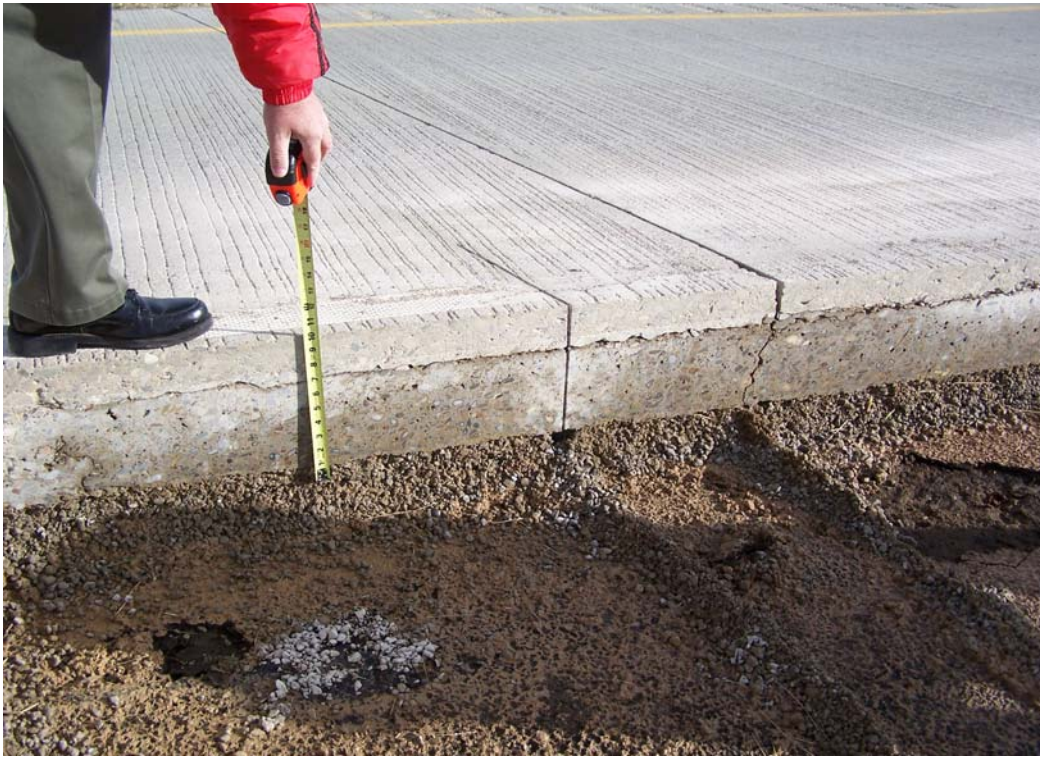
Photo 24 – Photo of longitudinal joint after concrete was removed.
