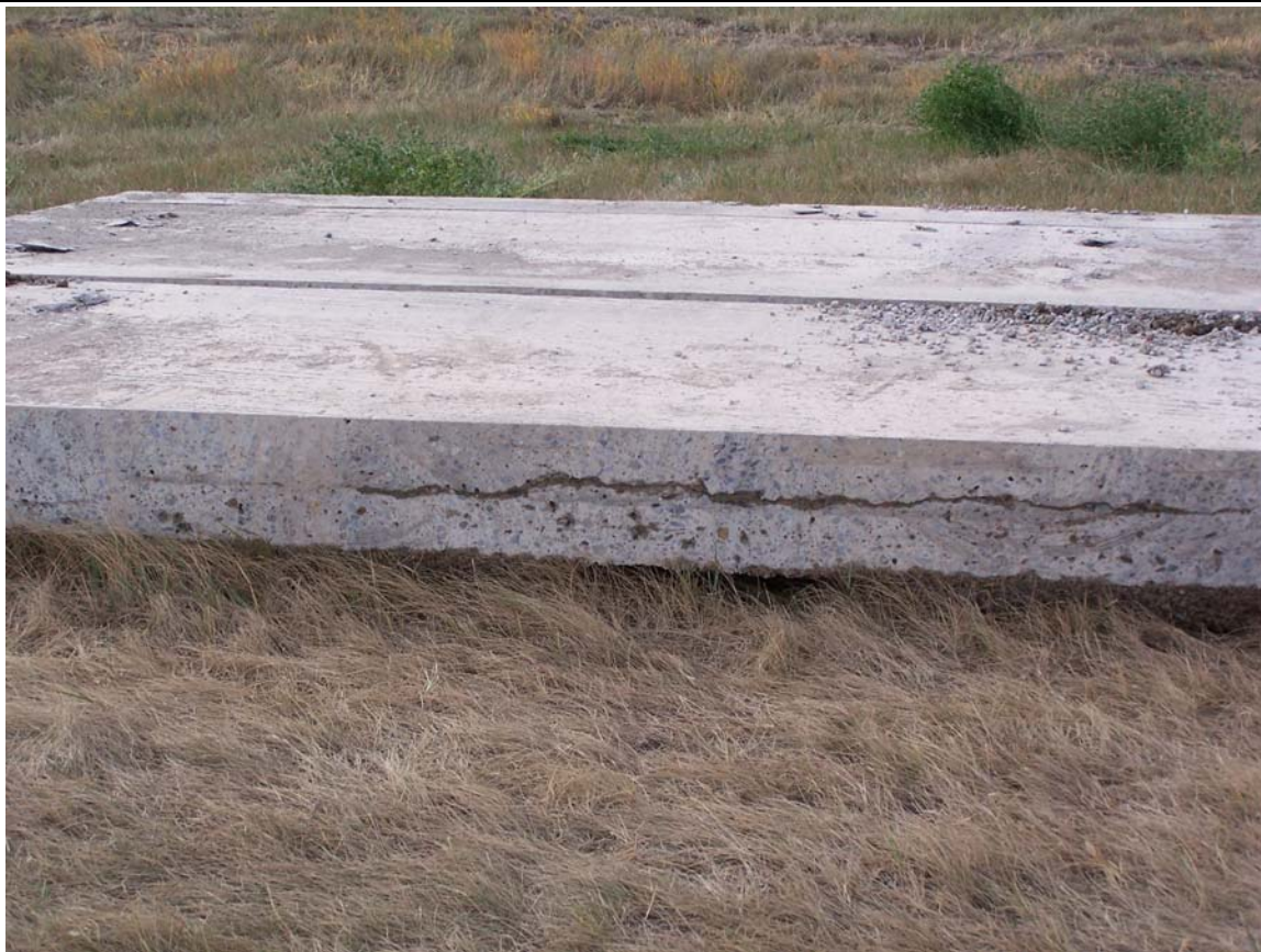
Photo 25 – Photo of crack running transversely in the center of a pavement section removed from roadway.
