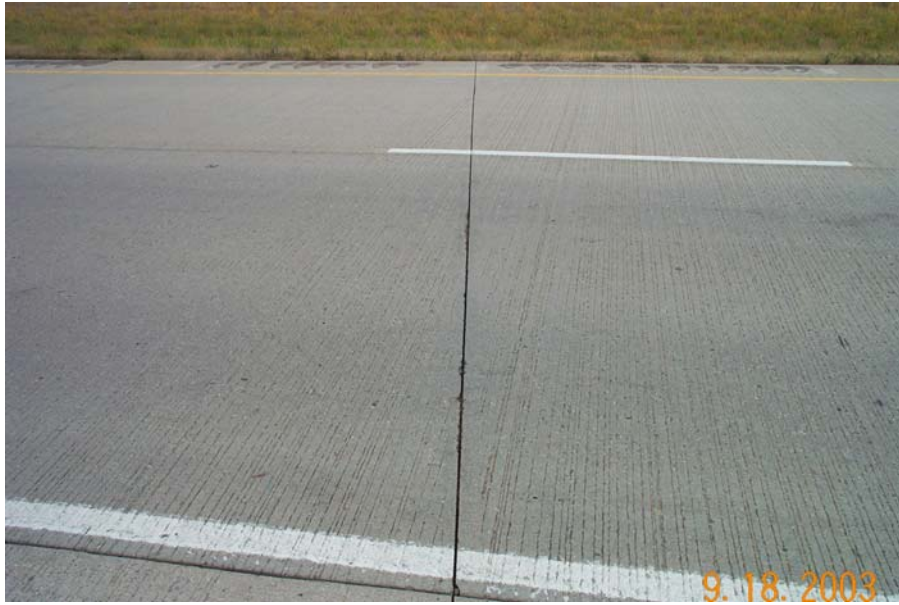
Photo 17 - Typical spalled joint in the test section.
