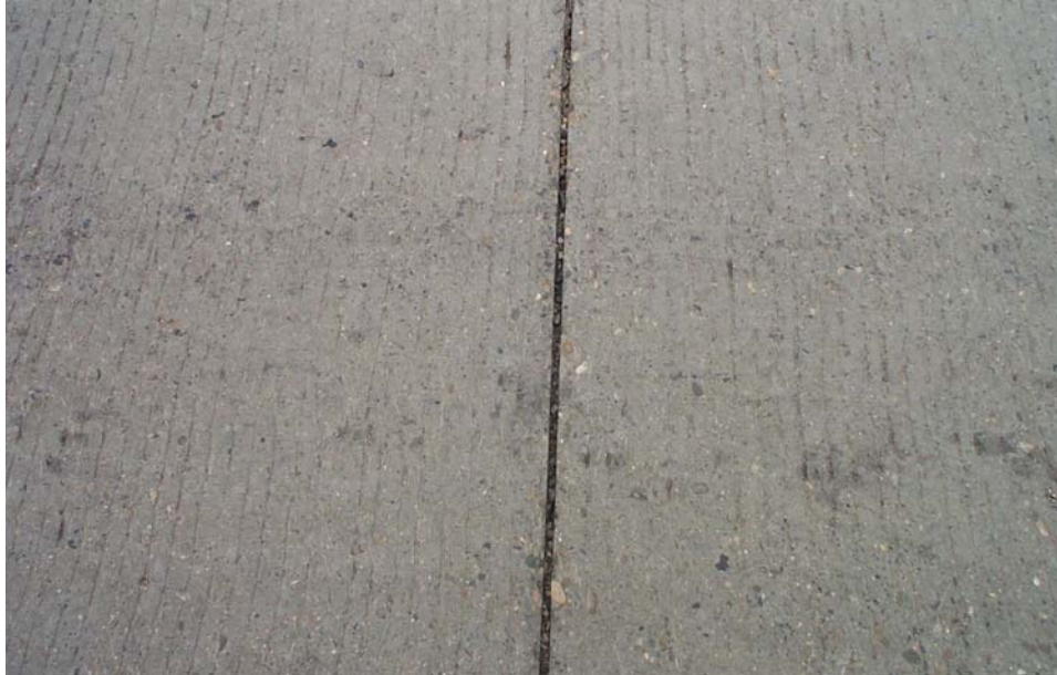
Photo 22 - Incompressible material in an unsealed joint at the shoulders.
