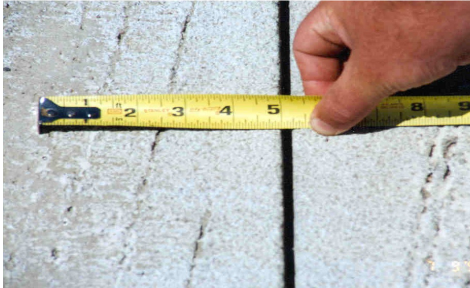
Photo 11 - Close-up view of a portion of an unsealed joint that was sawed correctly.
