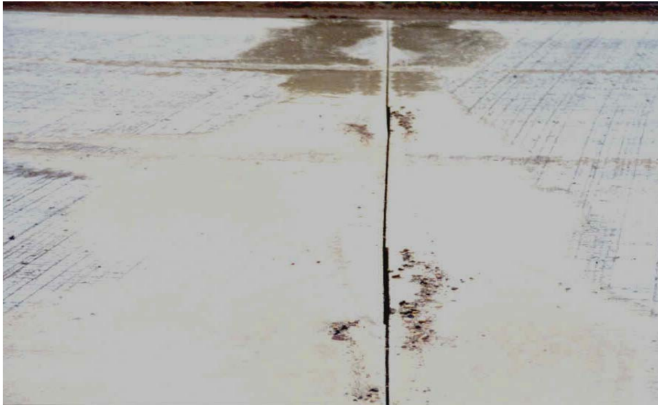
Photo 7 - Extra wide segment caused by the contractors gang saws being out of alignment.
