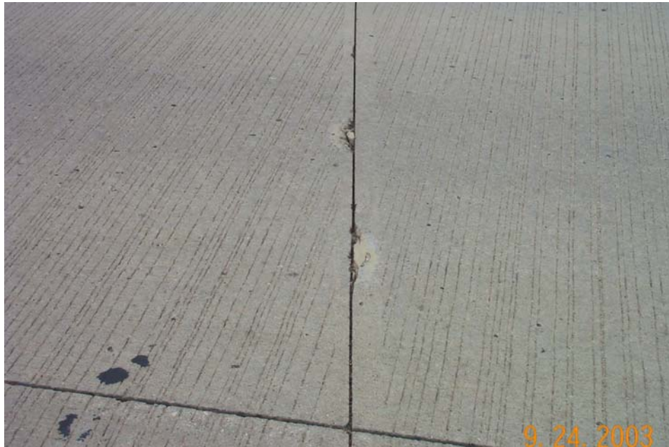
Photo 21 - Attempted spall repair in test section.
