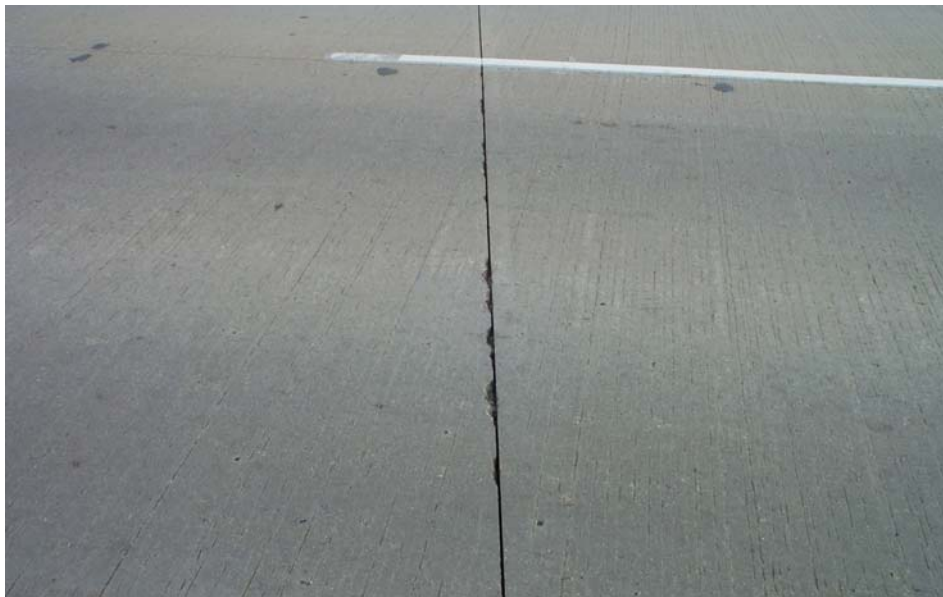
Photo 15 - Most severe spall in unsealed (test) section.
