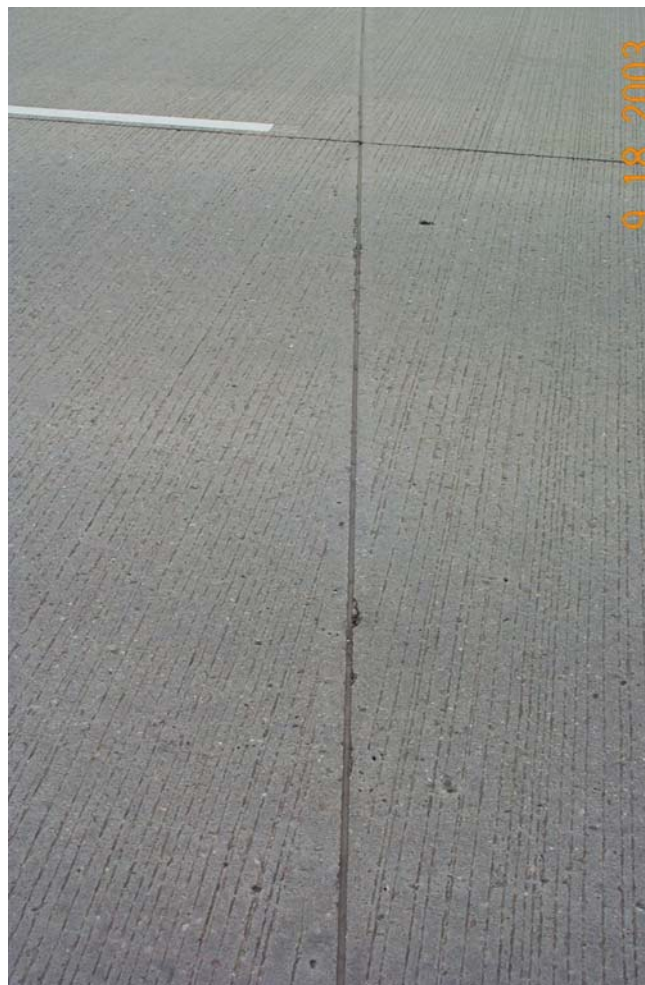
Photo 18 - Typical spalled joint in control section.
