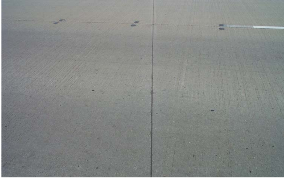
Photo 13 - Typical spalled joint in the sealed (control) section.
