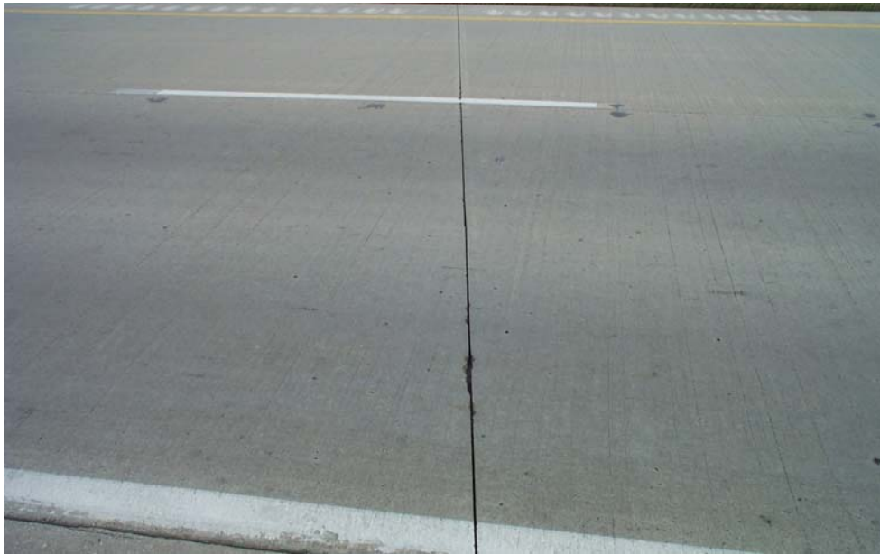
Photo 14 - Typical spalled joint in the unsealed (test) section.
