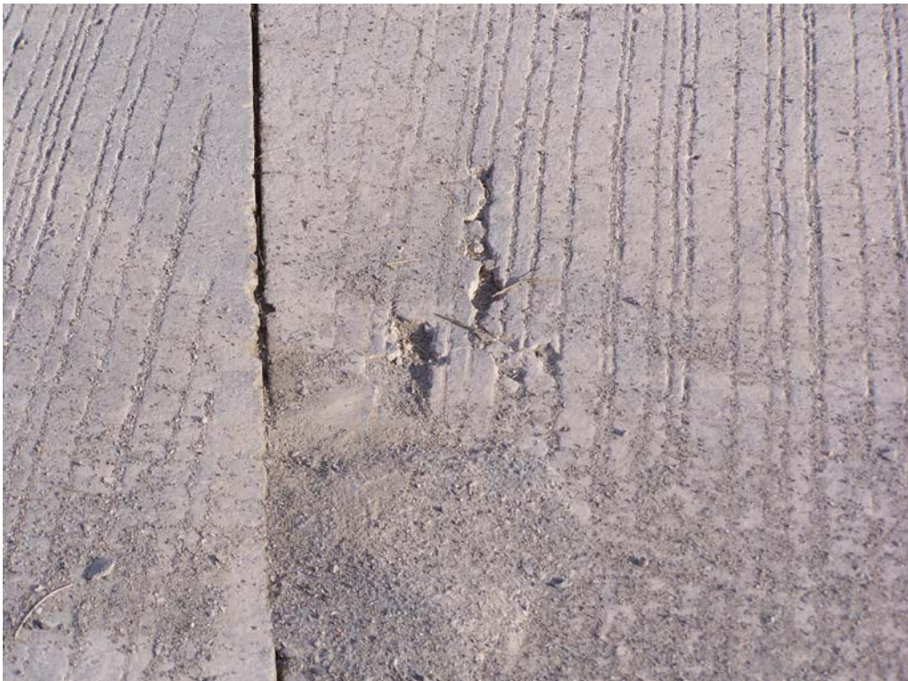
Photo 23 – Photo of severe map cracking next to transverse joint in “control section”.
