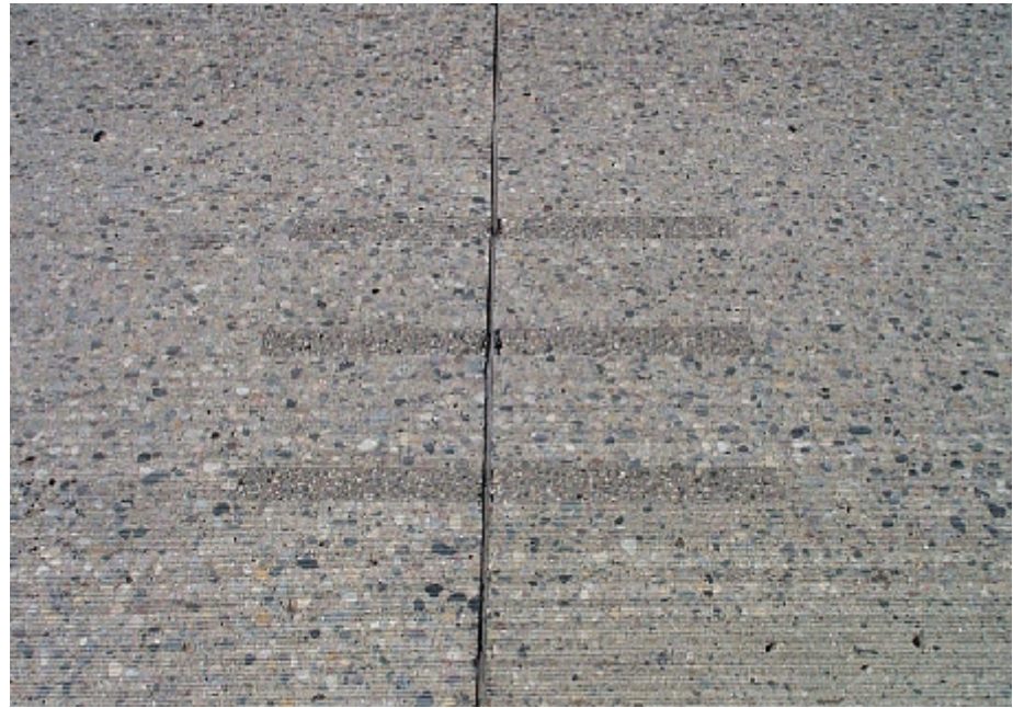
Photo 2. A view of a typical test joint where Steel bars were installed.
