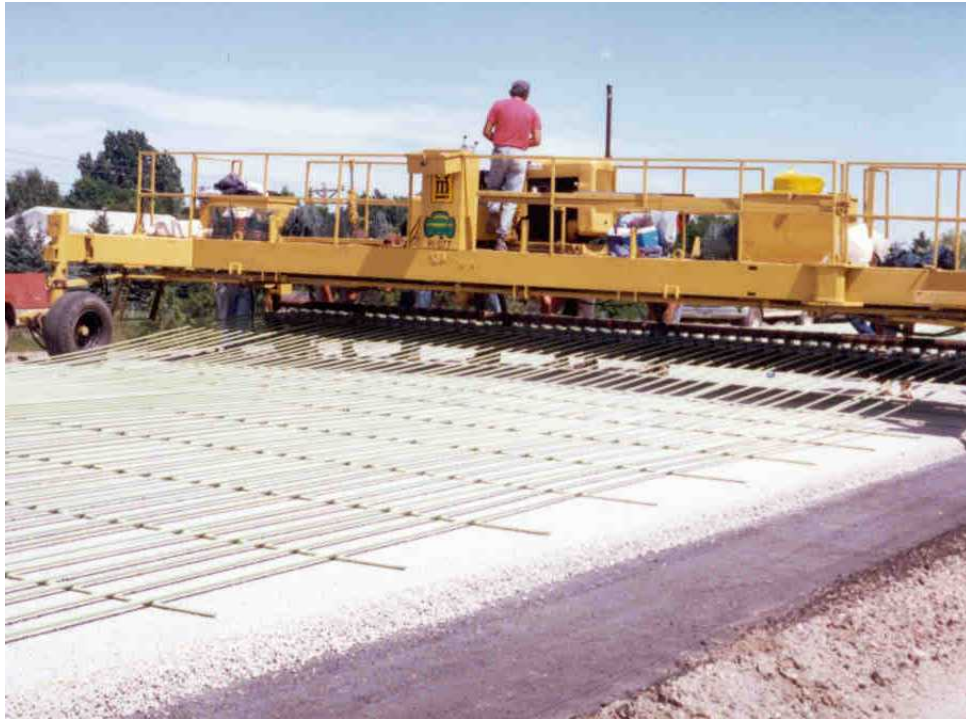
Photo 1 – Photo of the epoxy-coated reinforcing steel lying on top of the stabilized base.
