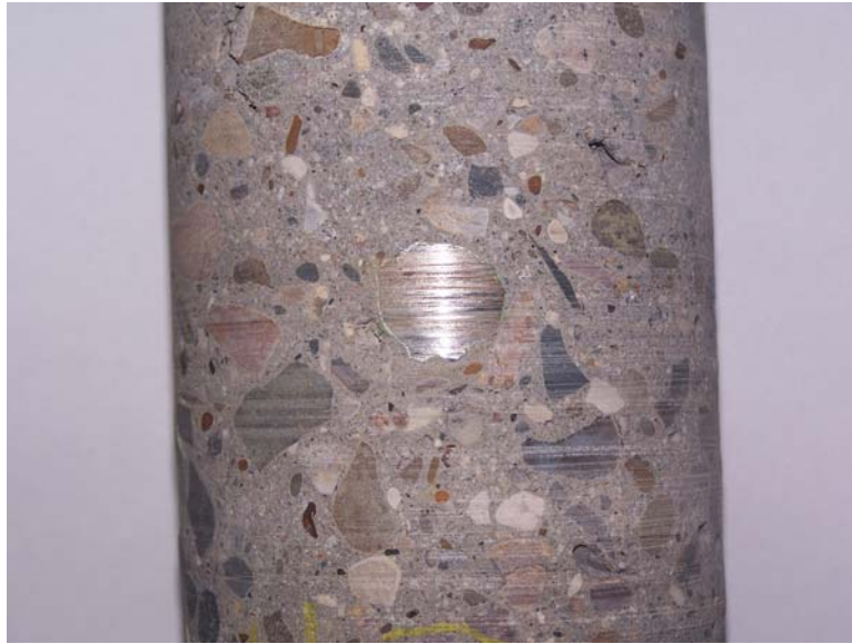
Photo 8 – Core containing epoxy coated reinforcing steel.
