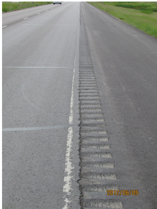
Photo 15: Damaged White Edge-line AWP with AW Elements
