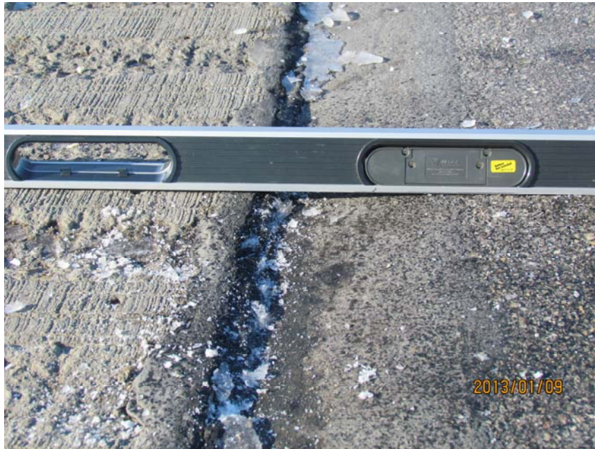
Photo 2 – Settling of the asphalt shoulders in Segment 2
