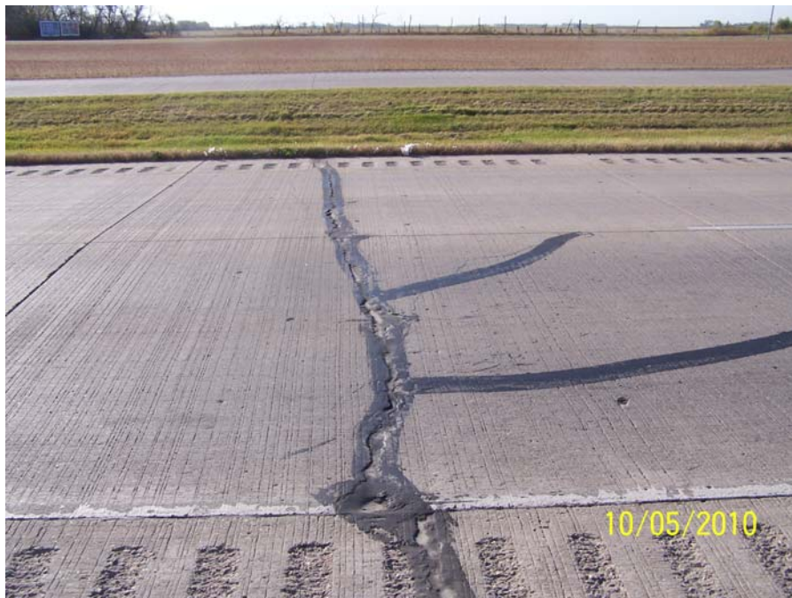
Photo 3: Distress located in Segment 3.
