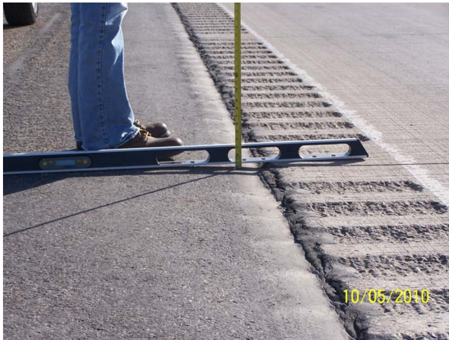
Photo 2 – Settling of the asphalt shoulders in Segment 2.
