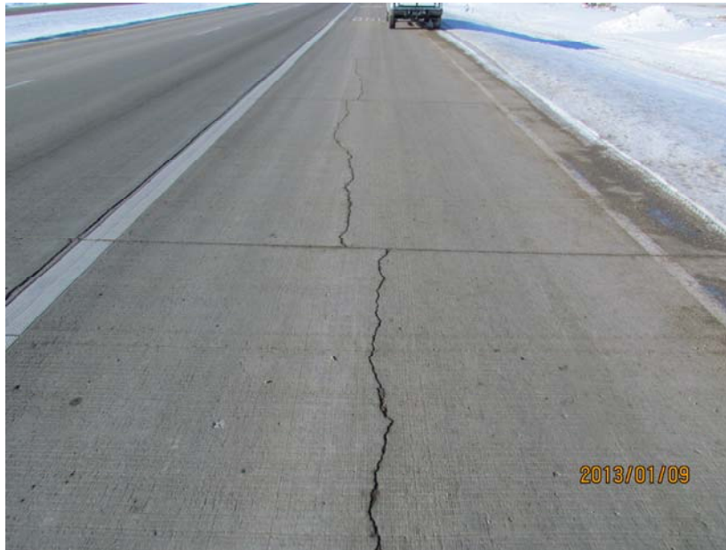
Photo 4 – Longitudinal crack in turning lane in Segment 3.
