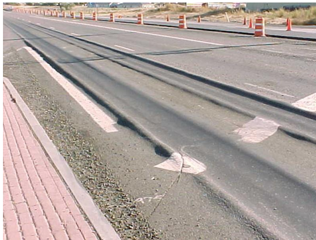
Figure 1. Rutting in a Two-lane Asphalt Pavement (Pavement Interactive, 2009)
