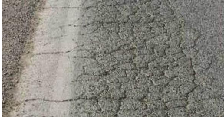
Figure 2. Images of Fatigue Cracking in Asphalt Pavement (Pavement Interactive, 2009)
