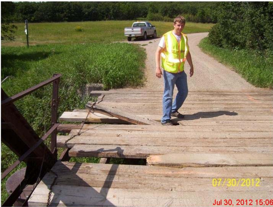
10-145-08.1 Broken Planks on Bridge Deck
