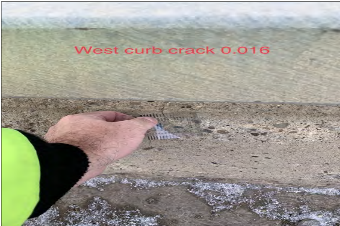
West curb crack .016
