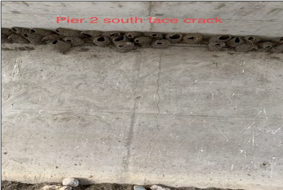
Pier 2 south face crack
