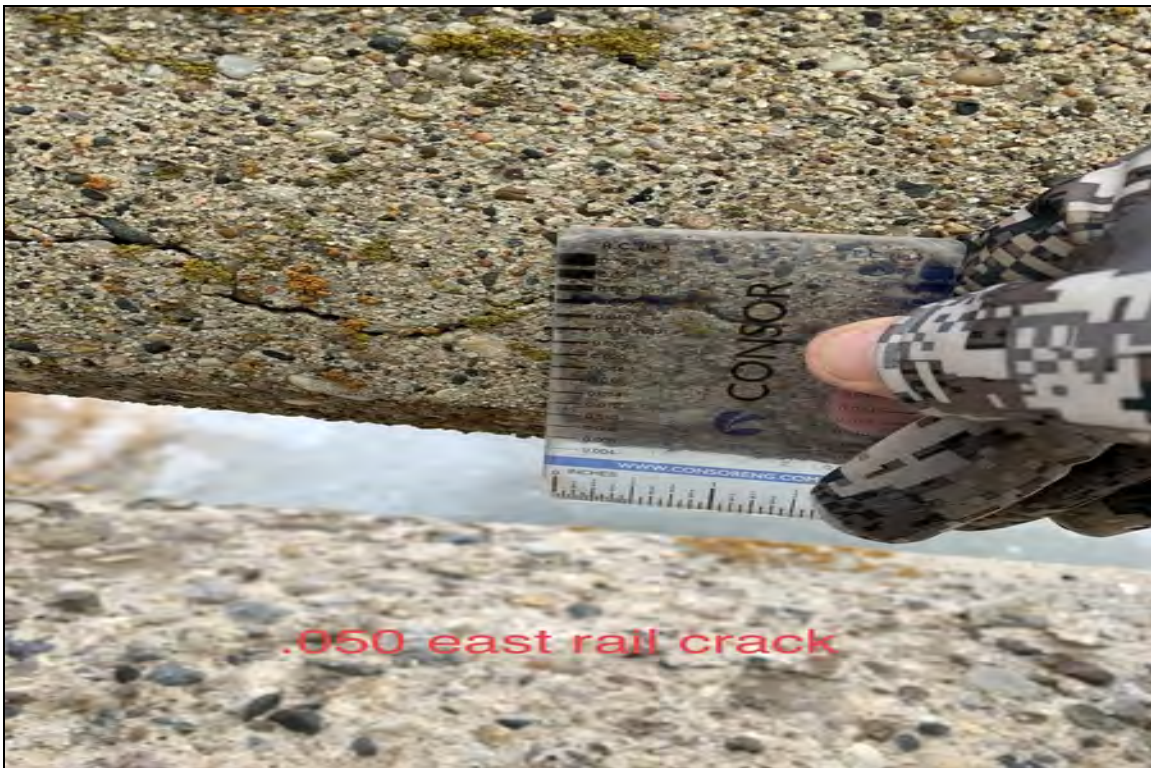
.050 east rail crack
