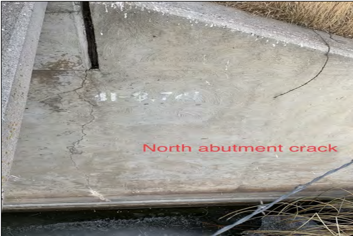
North abutment crack east end
