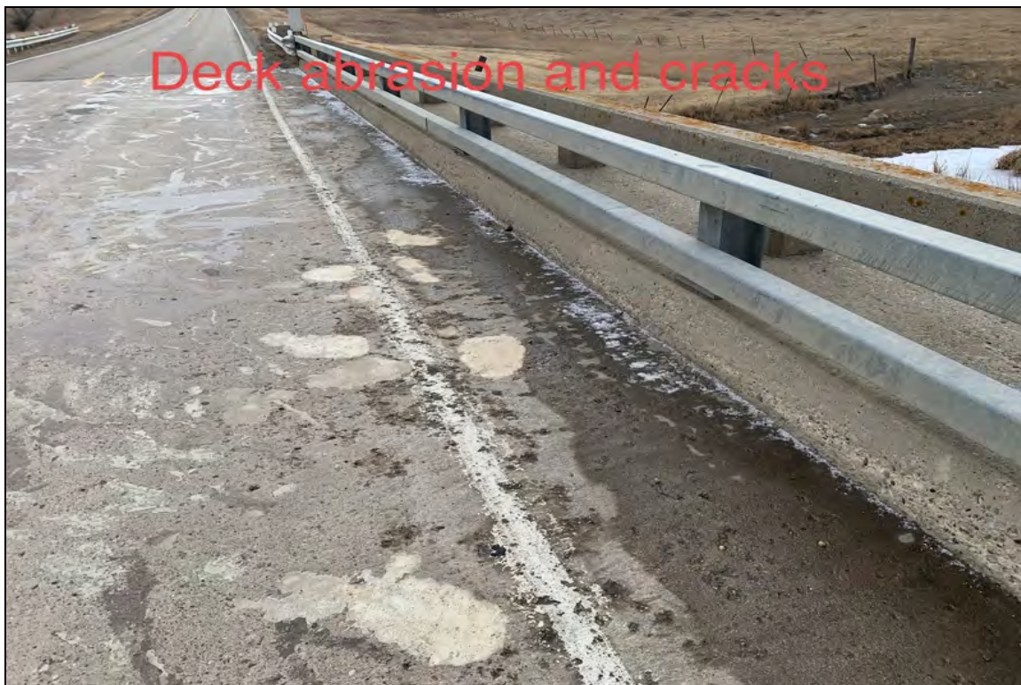
Deck abrasion and cracks
