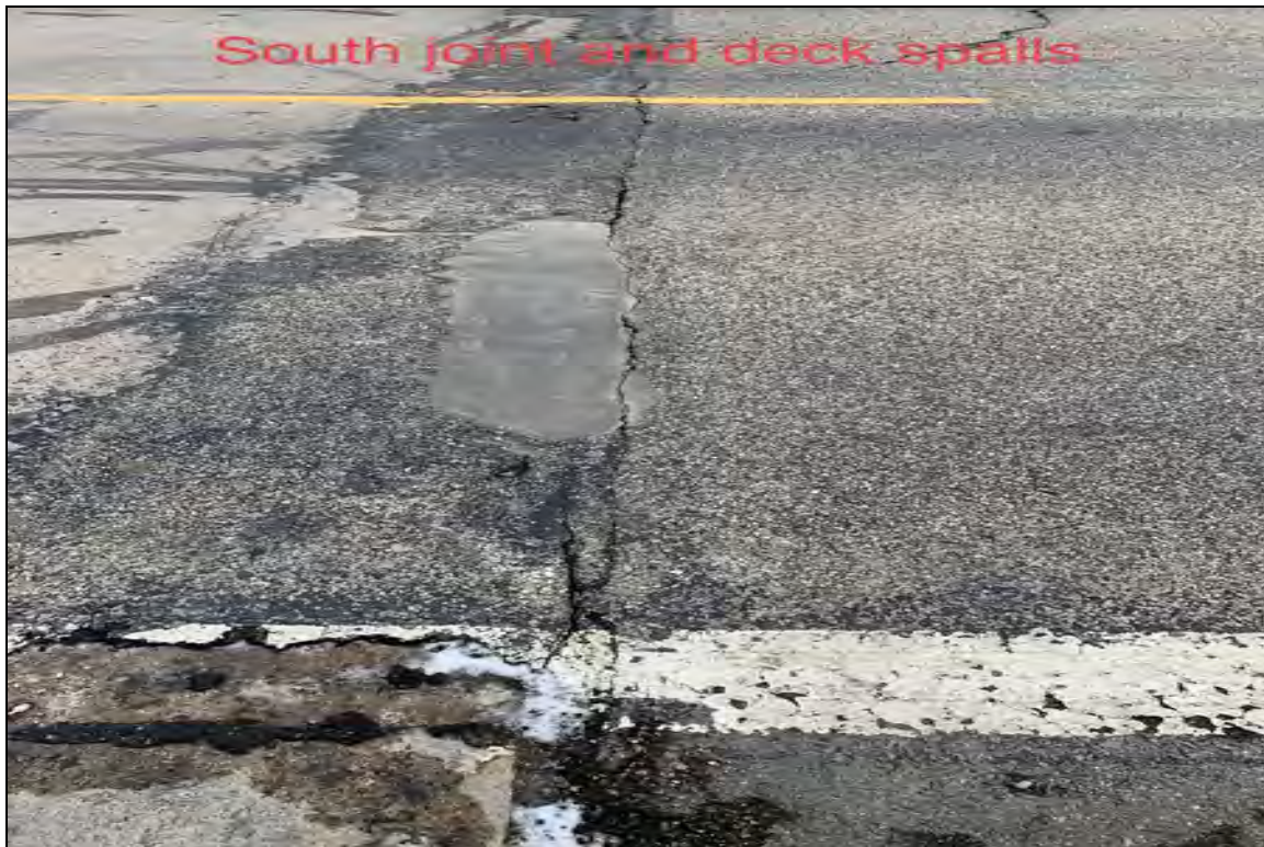
South joint and deck spalls
