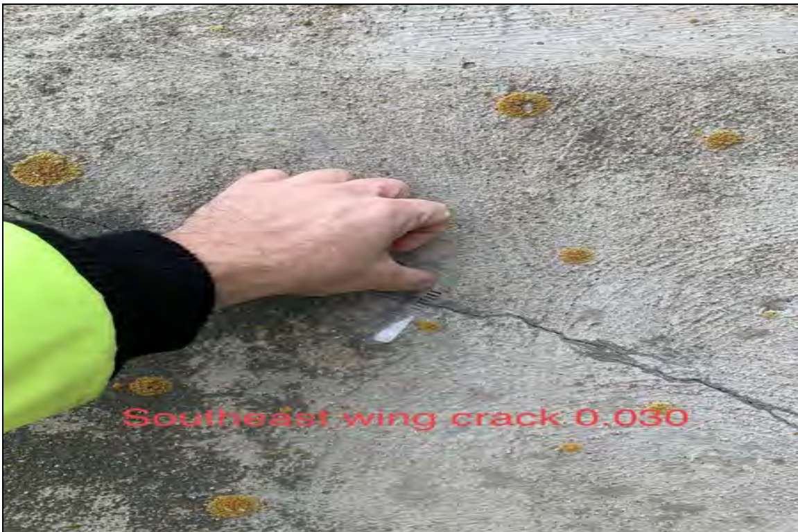
SE wing crack .030
