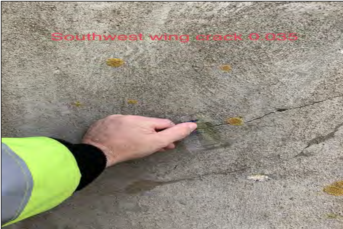
SW wing cracks .035
