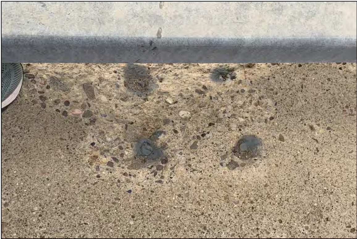
Old rail pedestal spot east rail
