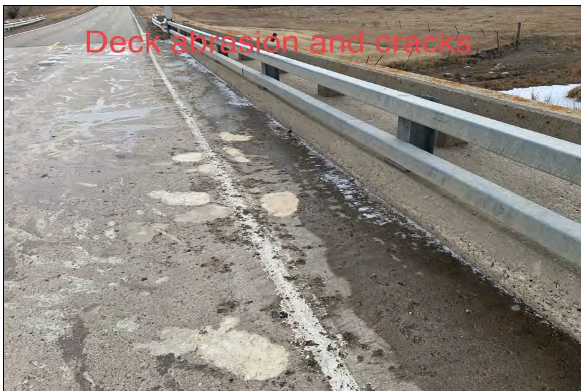
Deck abrasion and cracks
