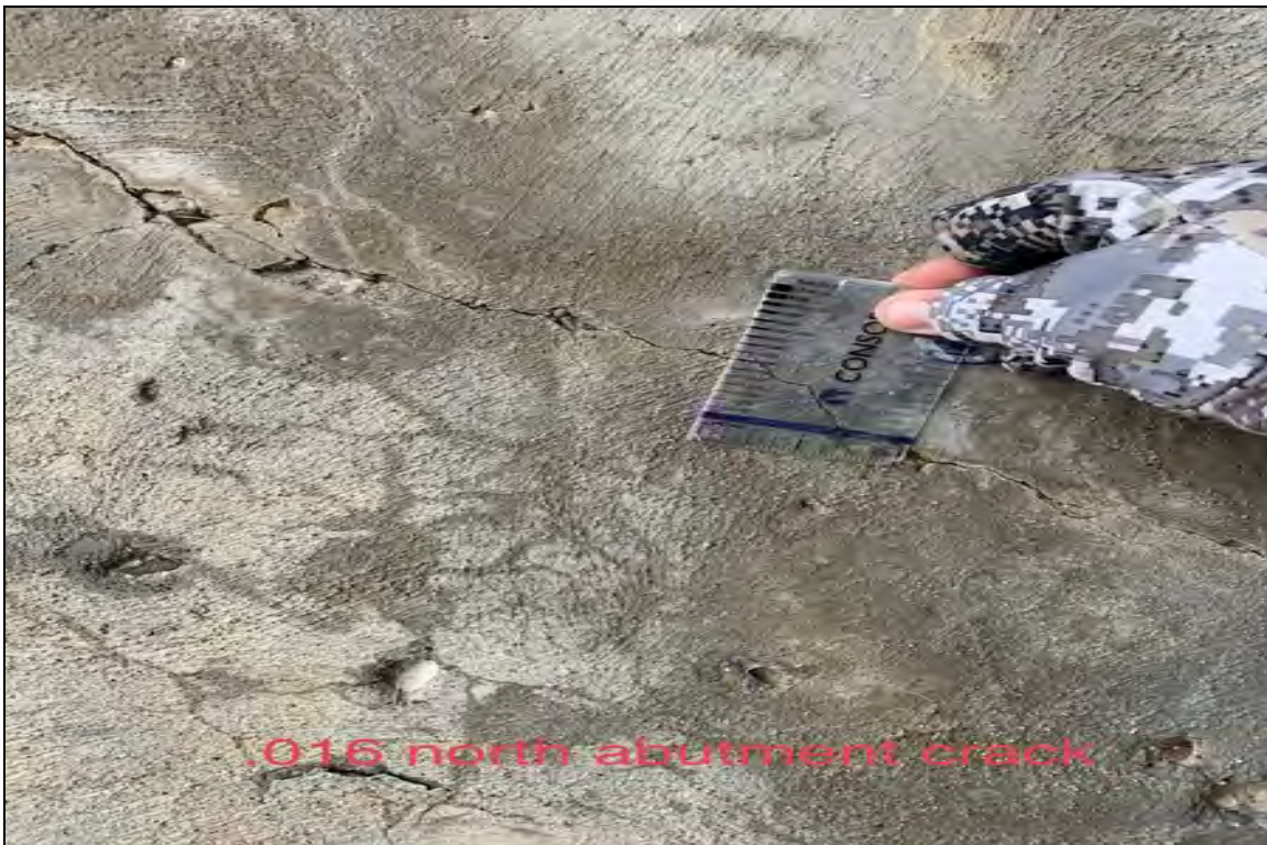
.016 north abutment crack
