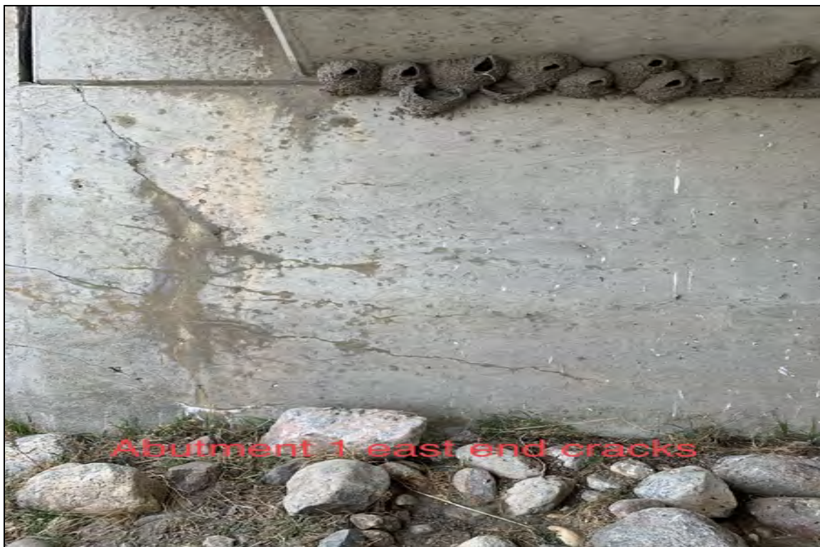
Abutment 1 east end cracks
