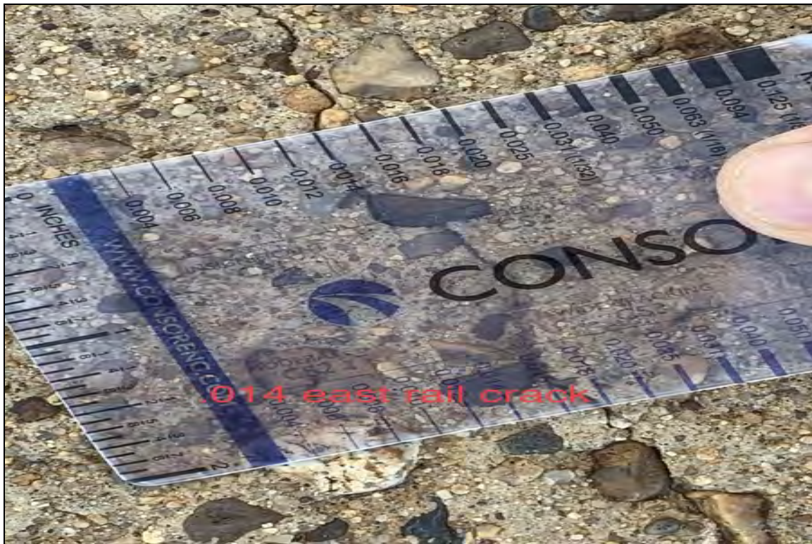
.014 east rail crack
