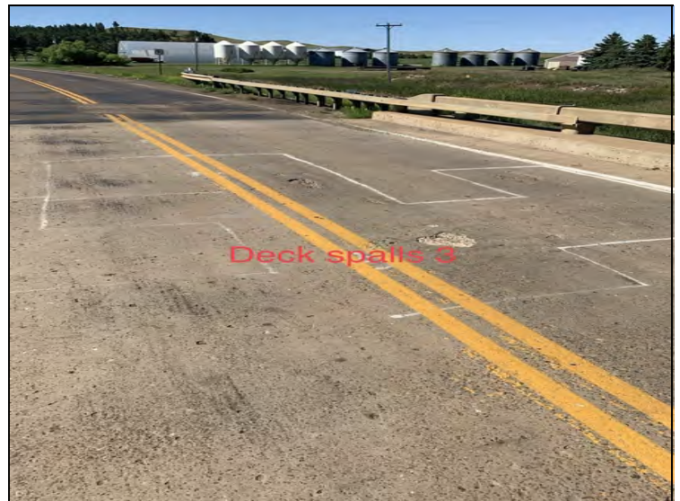
Deck spalls 3 spots
