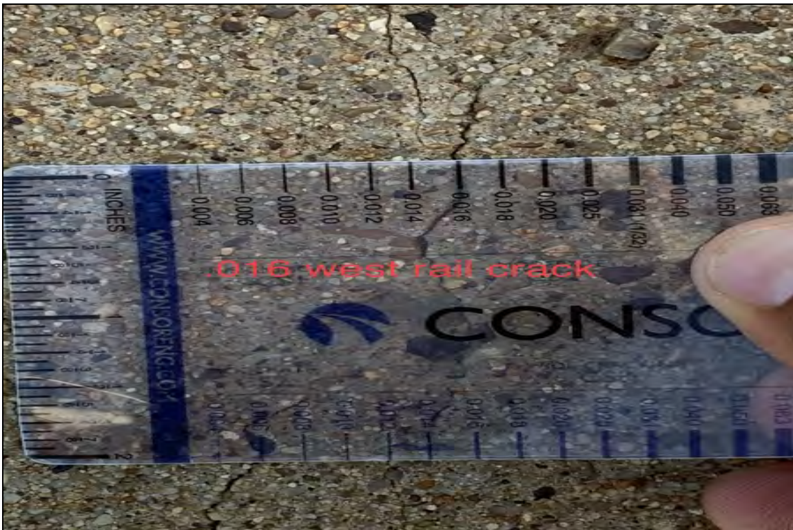
.016 west rail crack
