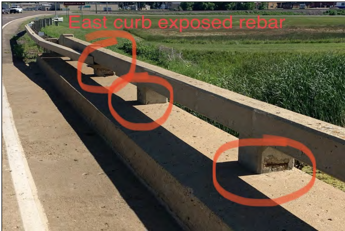
East curb exposed rebar on pedestals
