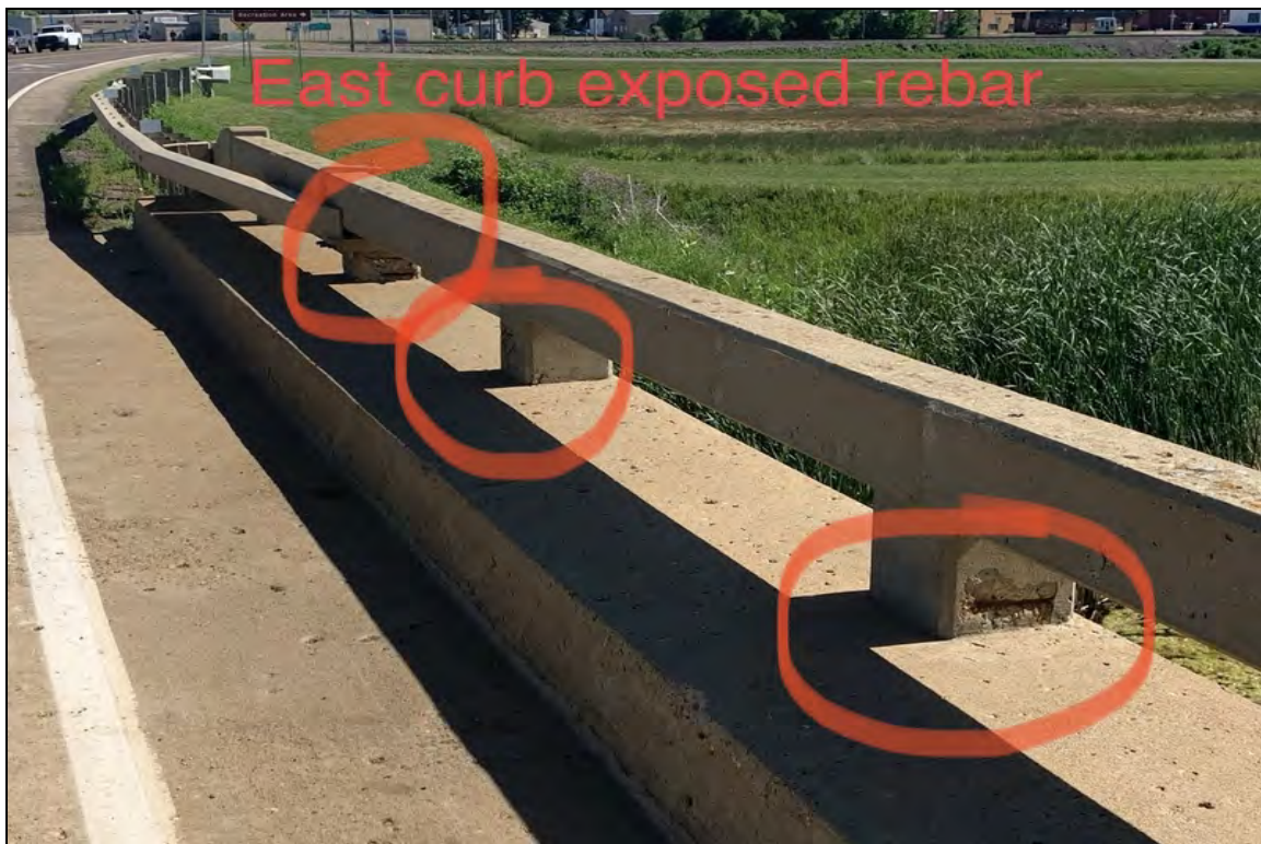
East curb exposed rebar on pedestals
