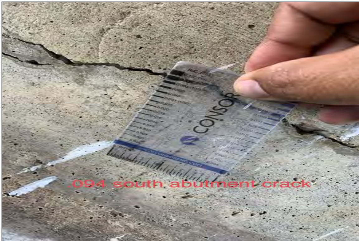
.094 south abutment crack horizontal
