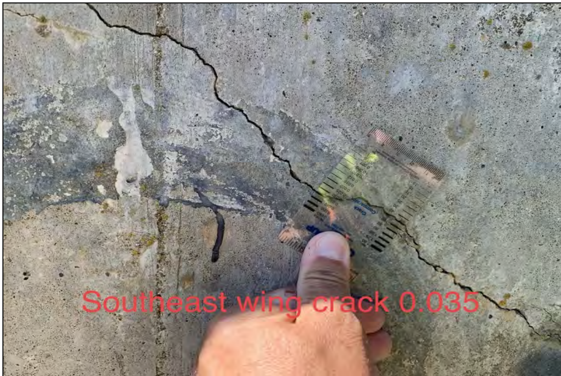
SE wing crack.035
