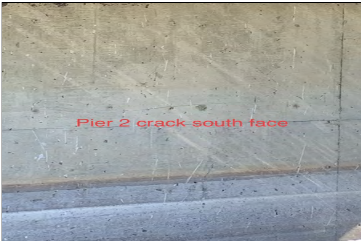
Pier 2 crack sout hface
