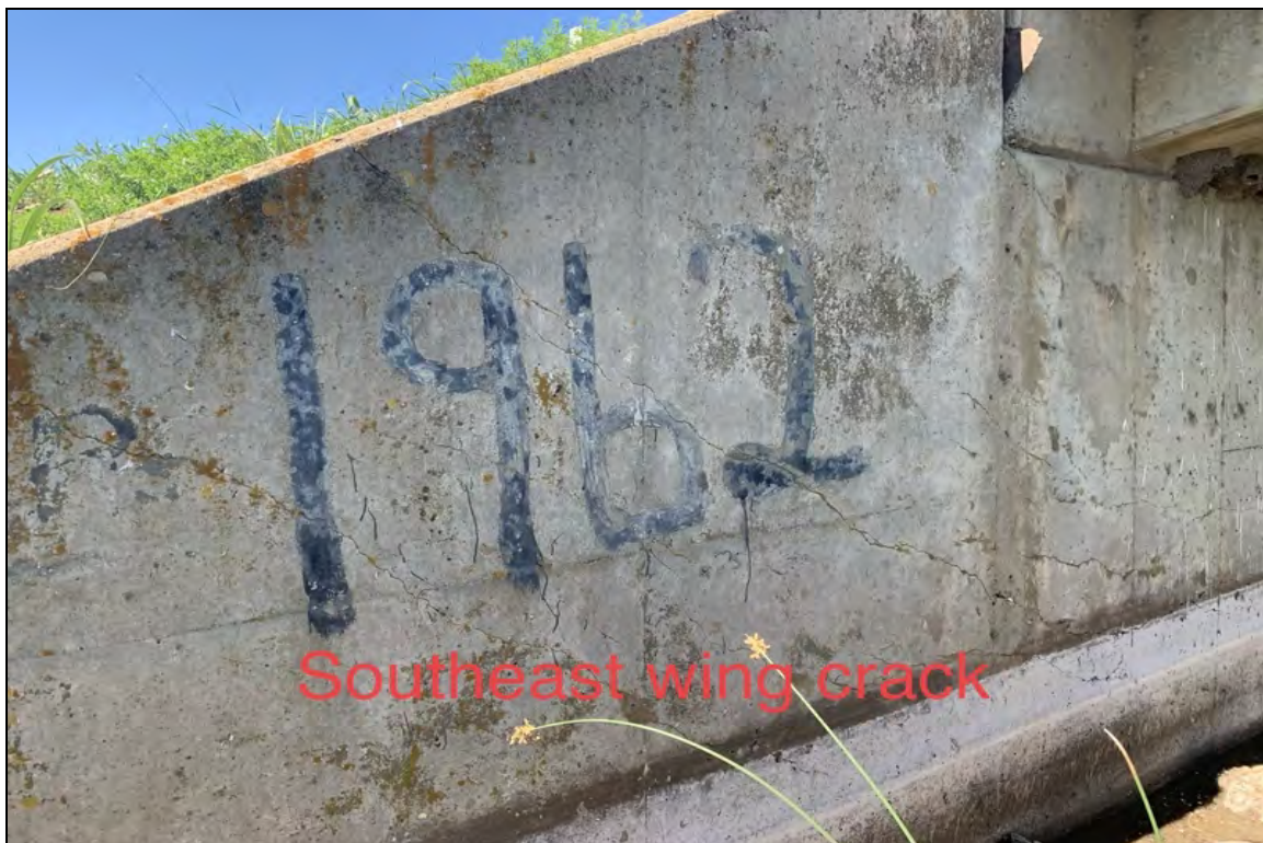
SE wing crack
