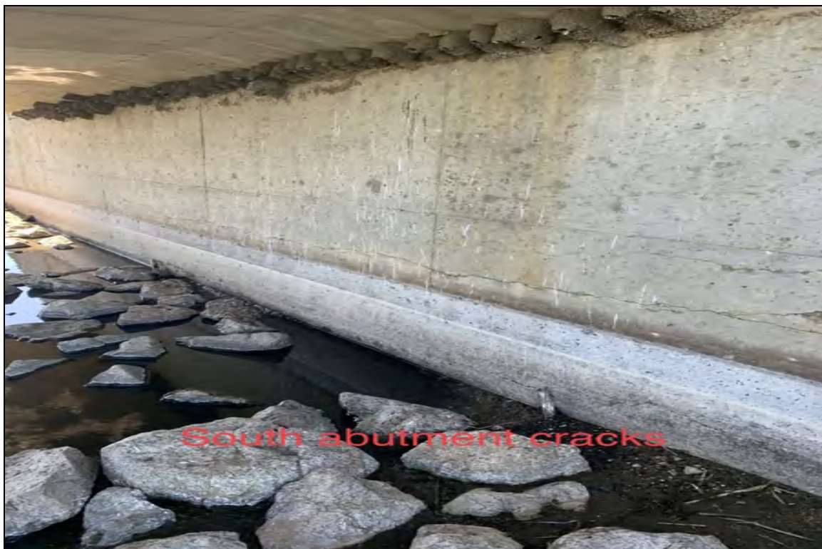
South abutment cracks
