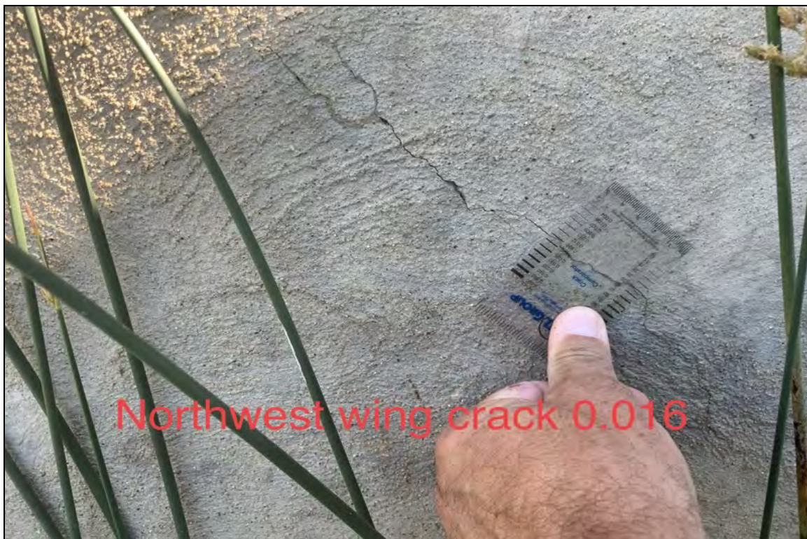
NW wing crack .016
