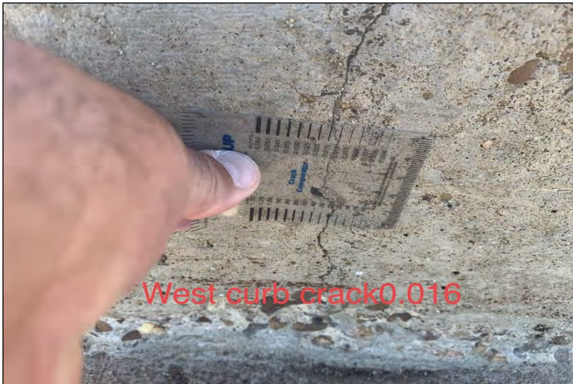
West curb crack .016
