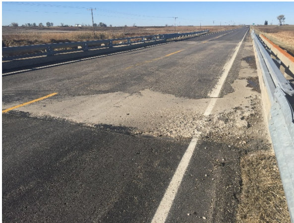
Figure 2 – Bridge Deck Deterioration
