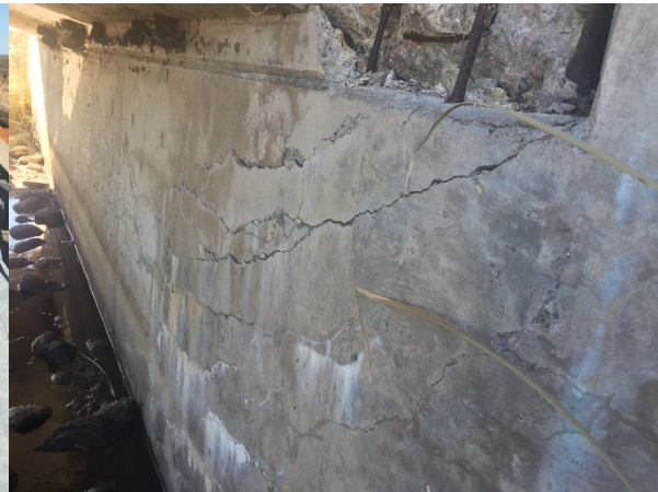
Figure 3 – Cracking at Abutments
