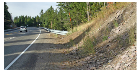
Photo C: Illustrates where the LON (minimum 75 ft. upstream of the area of concern criteria) was not met. A vehicle can potentially climb up the backslope, get behind the rail, and into the area of concern.
