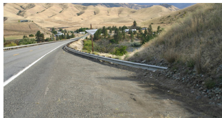
Photo B: Single Rail System - Foreslope MUST be 10:1 or flatter all the way to toe of backslope. If the backslope is flatter than 1:1, then the rail should be extended in front of the toe of backslope some distance (75') upstream of the area of concern before beginning the anchorage, as illustrated.
