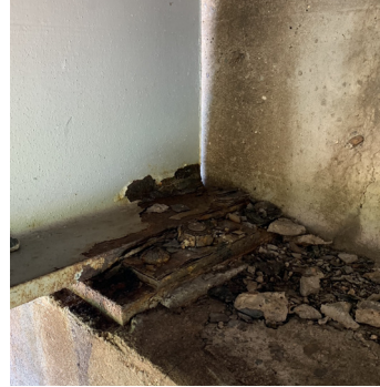
Girder/Bearing Corrosion and Abutment Cracking/Spalling at Bridge 24-000.320
