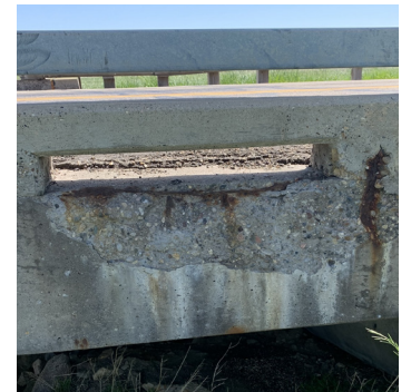
Concrete Girder Spalling with Exposed Rebar at Bridge 1806-035.070
