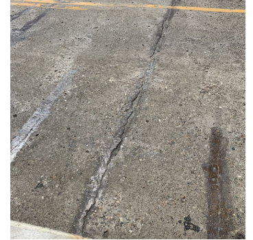
Deck Cracking at Bridge 24-000.320
