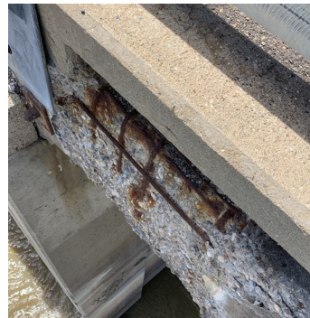
Concrete Girder Spalling with Exposed Rebar at Bridge 1806-034.280
