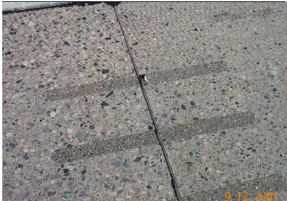
Photo 1. A view of a typical test joint where "Fiberdowel" bars were installed.
