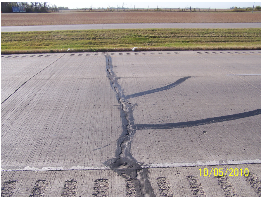
Photo 3: Distress located in Segment 3.
