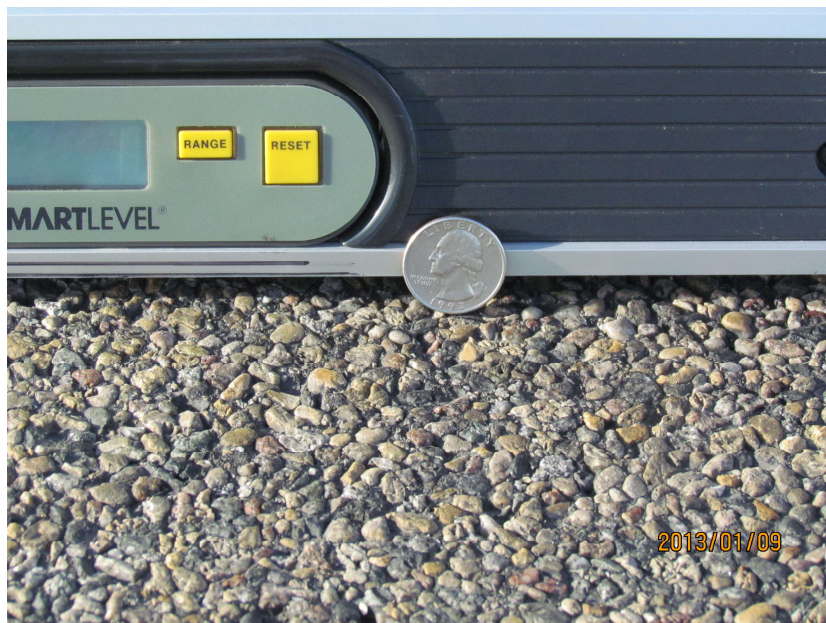
Photo 1: Rutting in a right wheel path in the driving lane of Segment 1.
