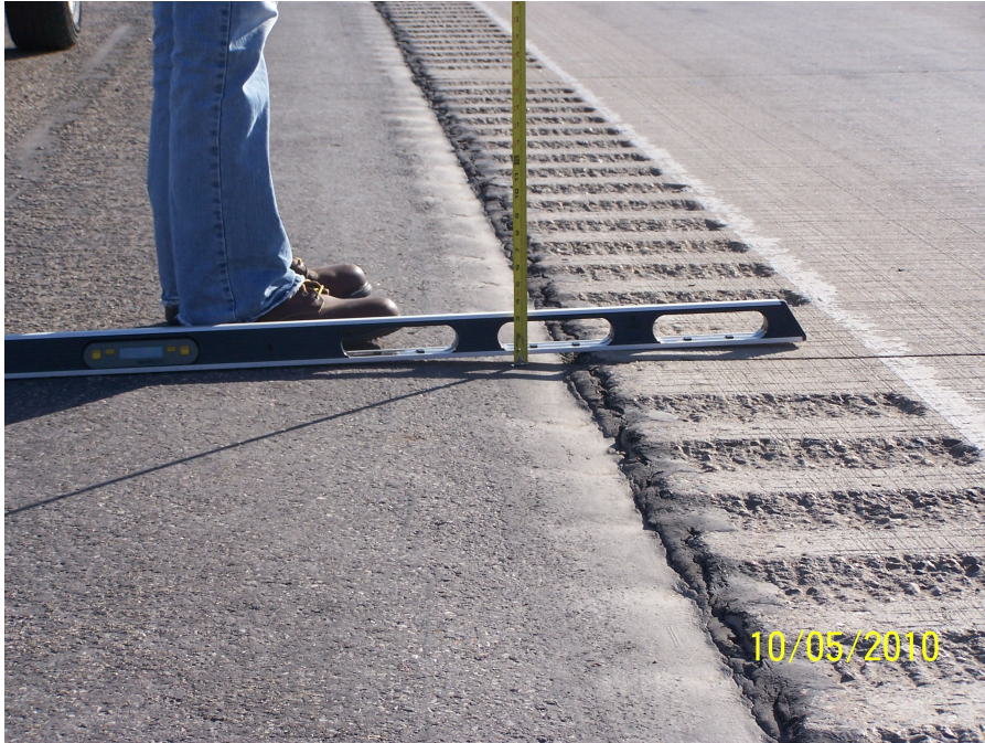
Photo 2 – Settling of the asphalt shoulders in Segment 2.
