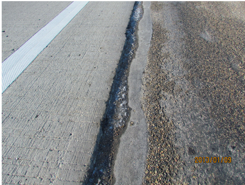
Photo 3 – Settling of the asphalt turning lane in Segment 2
