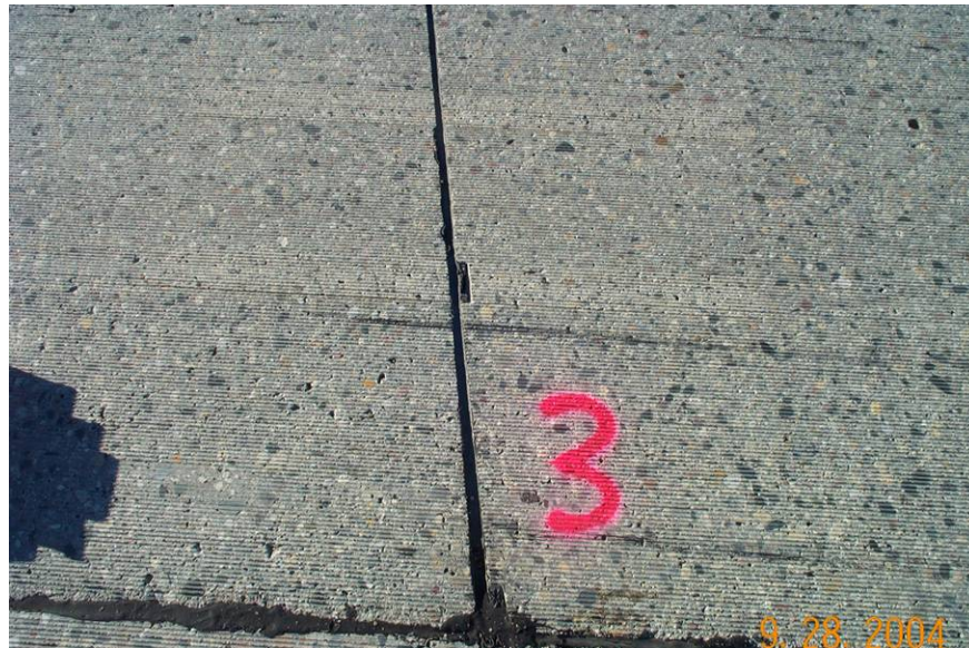
Photo 4 - Coreboard failure in control section 1.
