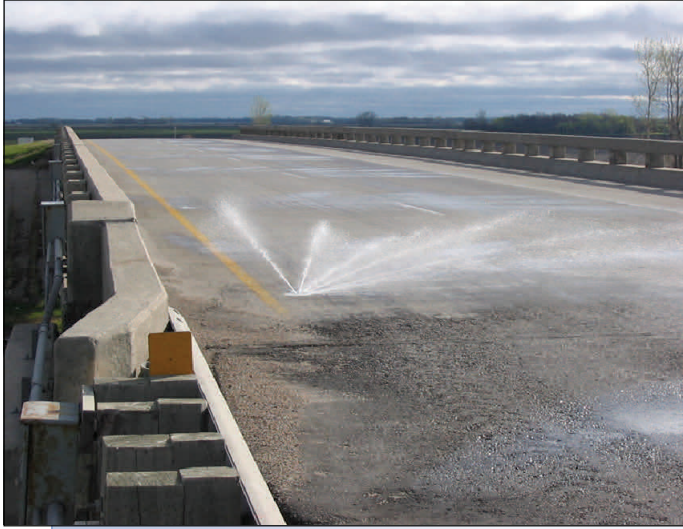
Spray disc in action on Interstate 29 Buxton Bridge south of Grand Forks, ND
