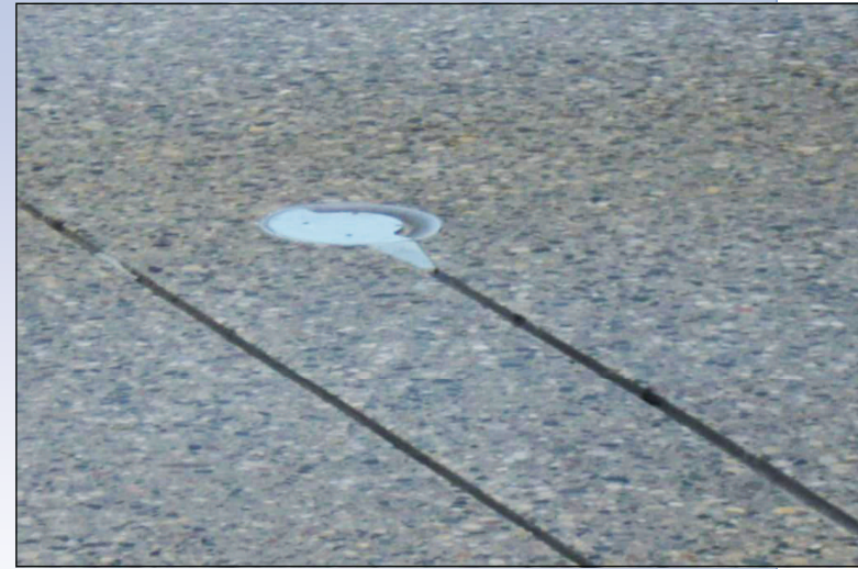
Spray disc on Interstate 94 Red River Bridge between Fargo, ND and Moorhead, MN
