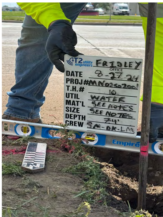
Photo No. 3 Board Photo
