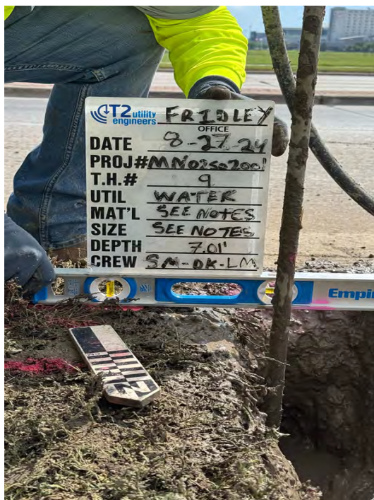
Photo No. 3 Board Photo
