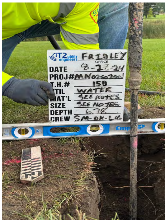
Photo No. 3 Board Photo
