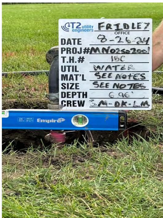
Photo No. 3 Board Photo
