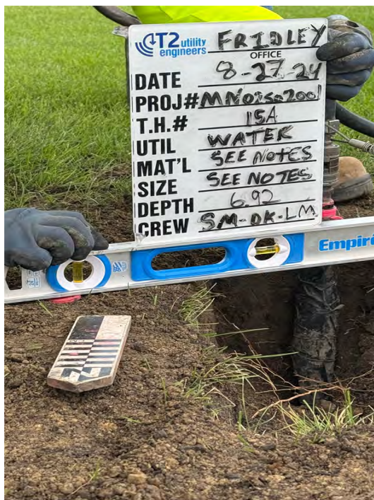
Photo No. 3 Board Photo
